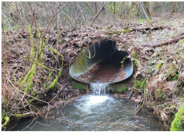
Before: Old culvert blocking fish passage on a tributary to Cheney Creek. Photo by Luke Wimmer, Applegate Partnership.
